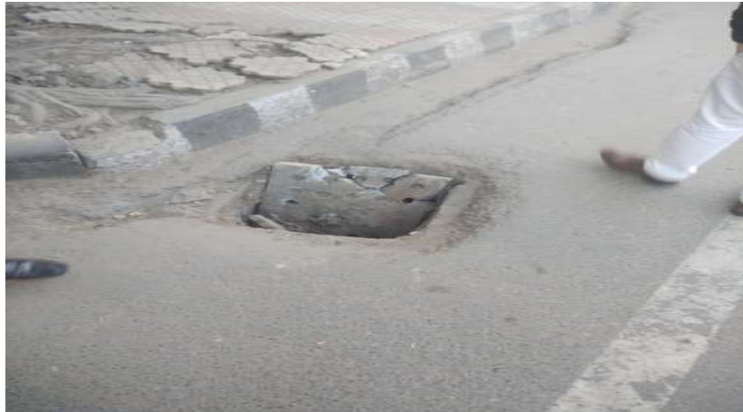
Image showing broken and unattended manhole and walkpath near Nagar Nigam
